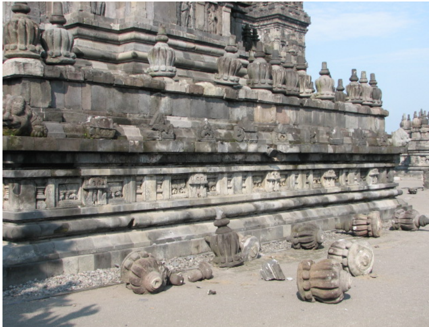
The damage occurred in Nandi Temple (Photo courtesy of BP3 DIY)
